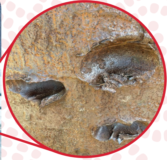
Close up of the pillbox at Memorial 39-45 showing damage from enemy artillery.
