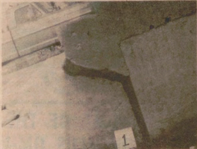
Front step of Mr. McIvor's house. No sign of steel reinforcement.
