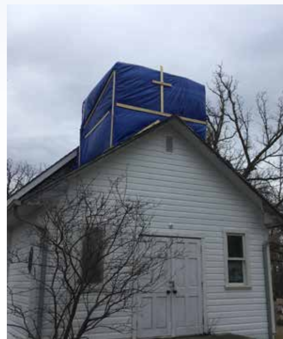
The new vestibule will be historically correct and represent the earliest foyer and steeple as closely as possible.
